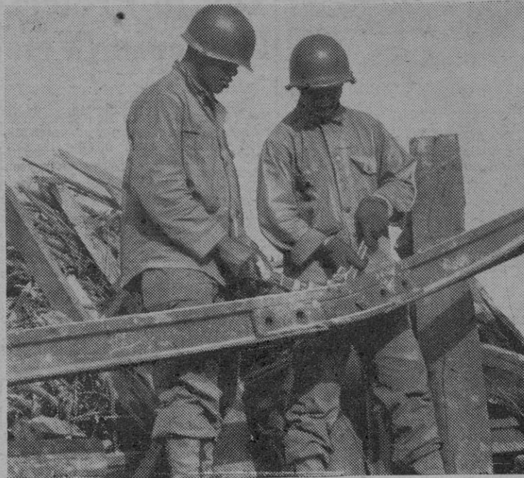
Men from the 392nd Engr. Regt. salvage old rails, ties and other track material used in extending the rear transportation network to forward echelon railheads.
