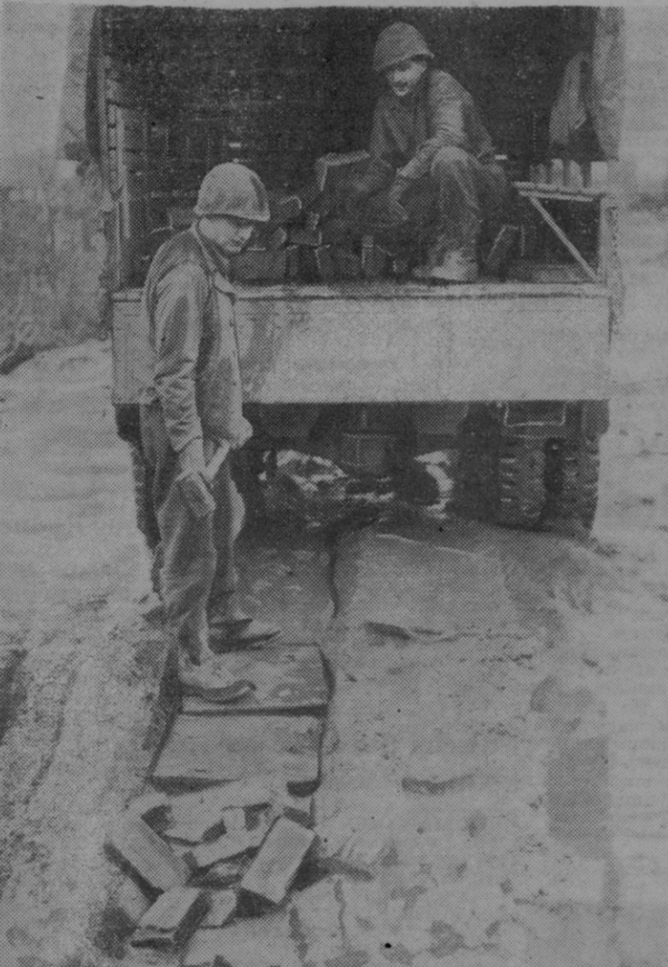
Traffic was bogged down by mud, so Pvt. Ray Shaffer, with sledge, and Pvt. Edward Capazi, engineers of the 102d Div., were forced to fill mudholes to keep the traffic rolling at Ubach, Germany.
