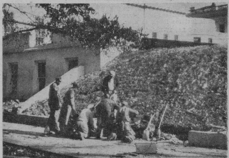
NEW WING STARTED: Workmen remove the stone base along the grounds at the western side of the White House in preparation for an addition to the executive offices. Work is proceeding, although the Senate has rejected President Truman's request for 870,000 dollars for the project.
