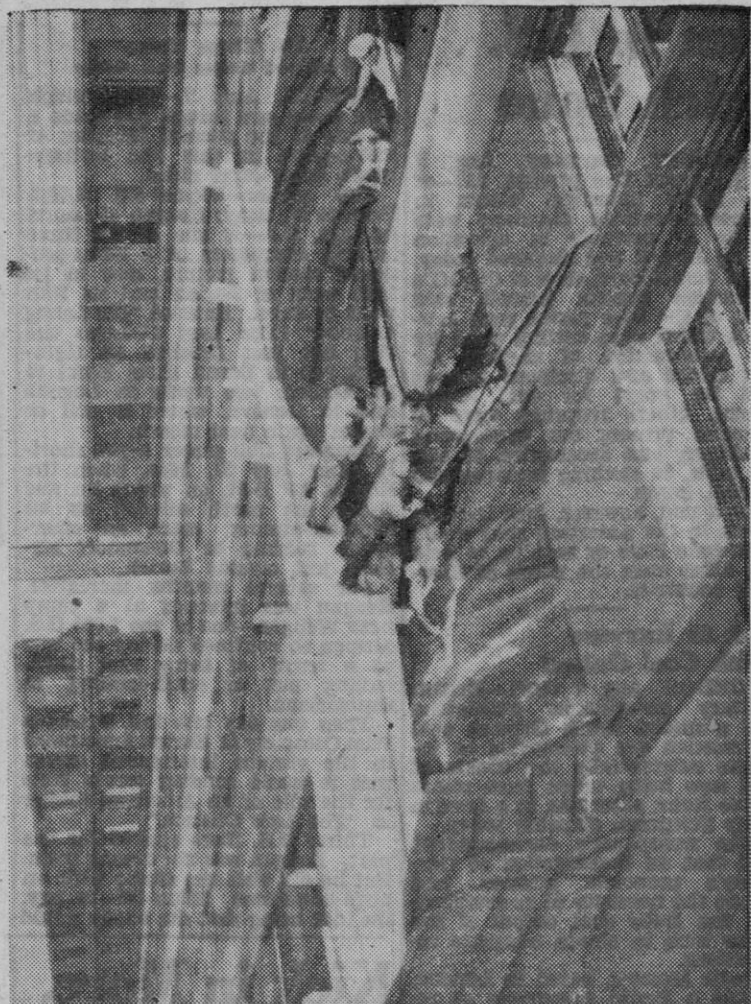
Workmen on ledges and scaffolding between the 78th and 79th floors clear away debris to begin repairs on the Manhattan skyscraper.
