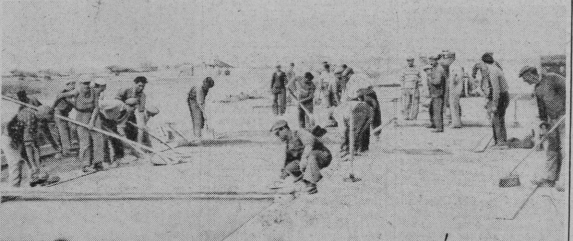
French workmen smooth the fresh concrete on one of the new runways at Orly Field near Paris. Present plans call for construction to make Orly one of the most modern airfields in the world.
