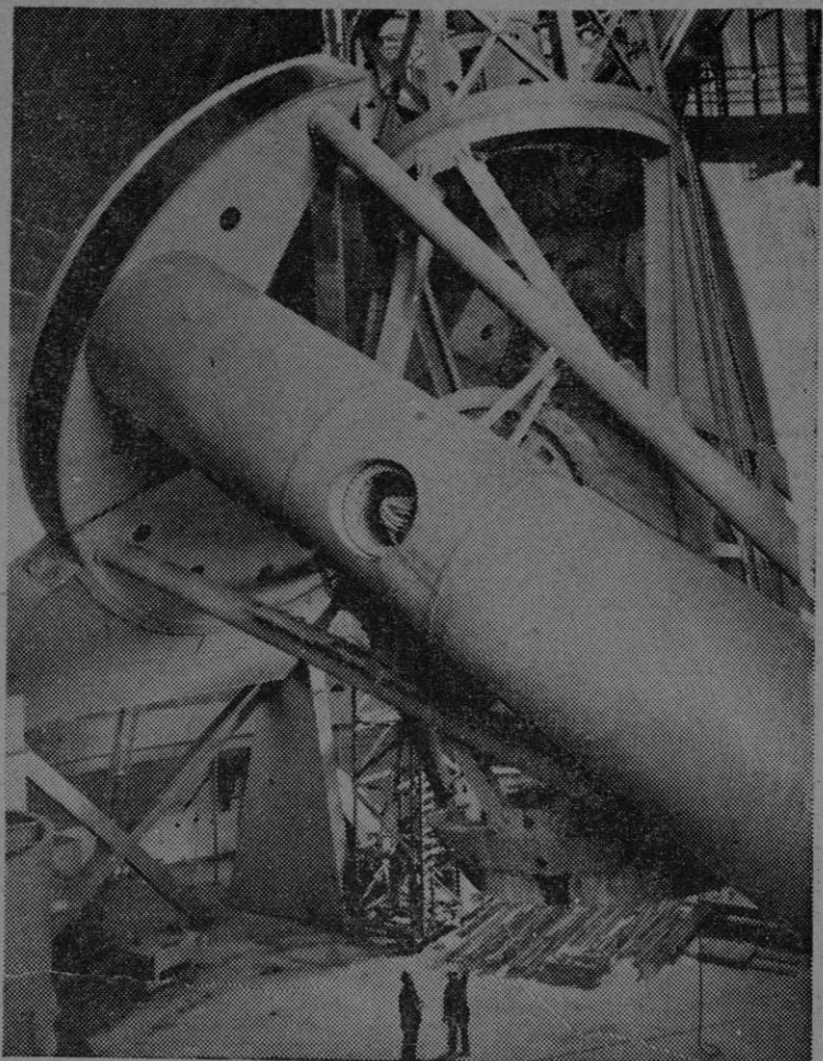
Work has been resumed on the world's largest telescope atop Mt. Palomar near San Diego after delays due to the war. The delicately balanced mechanism, weighing about 500 tons, is nearly complete, but the 200-inch mirror will not be ready for at least another year.
