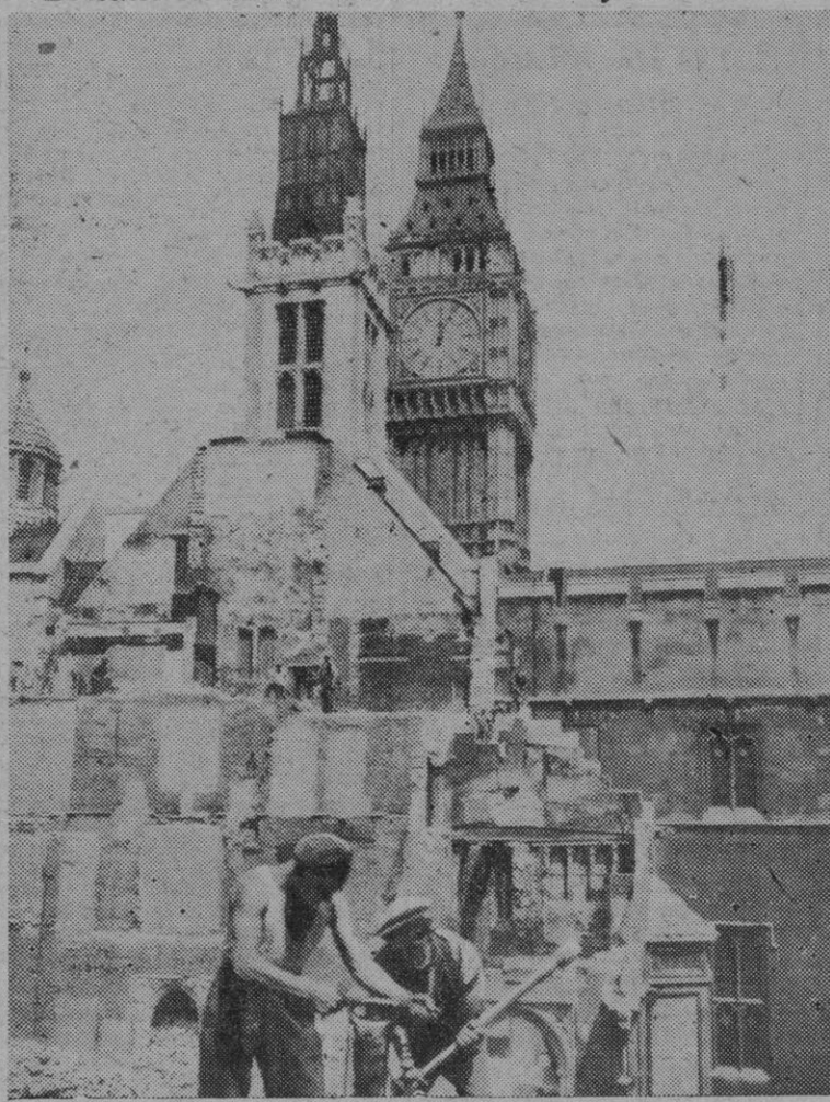
British workmen tear down a section of the House of Commons wall destroyed in the 1941 blitz. After the site is cleared, work will begin on a new building. London's famous Big Ben is in the background.
