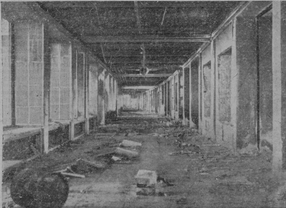
This is the way one of the corridors at Tempelhof looked when the ATC cadre arrived. It was described as one of the cleaner ones.
