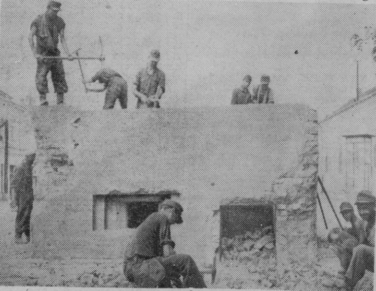
German PWs in St. Pazonva, Yugoslavia, demolish a pillbox built by Nazi occupation forces as part of the Wehrmacht's defense system.
