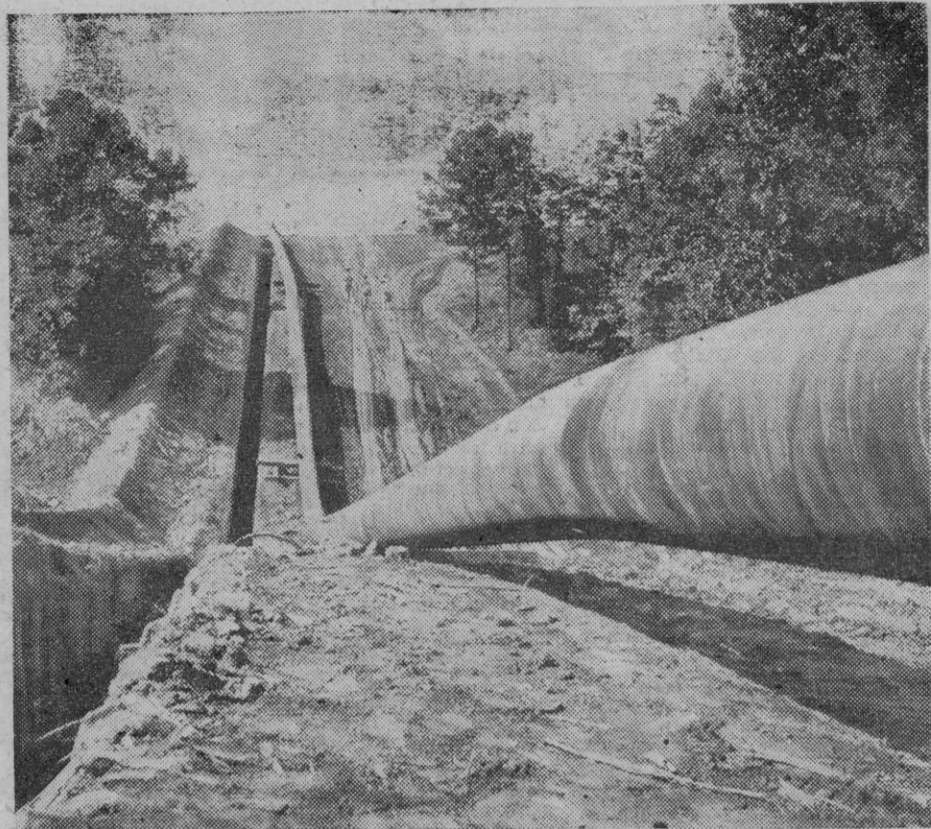
Wide World Resembling a giant worm, section of "Big Inch" pipeline is shown in early construction stage. Completed line now speeds war-needed oil from Texas to Atlantic seaboard.
