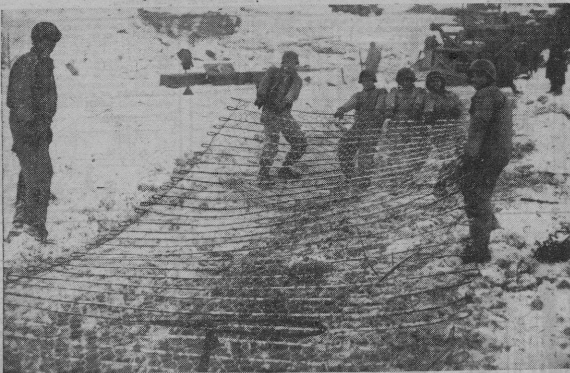
Engineers of the U.S. First Army are constructing a temporary road leading to a bridge somewhere in the battle-zone in Belgium. They're hauling up wire netting over which supply convoys will soon be rolling.
