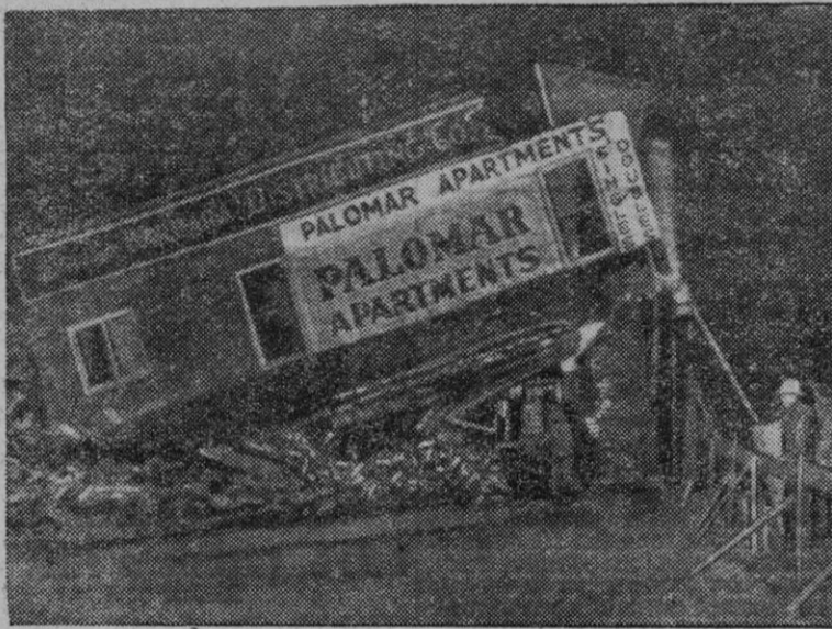
A soft-drink bottling plant in downtown Santa Barbara, Calif., was demolished recently in an explosion and fire. The mishap occurred when a truck driver stepped on the starter of a car containing butane gas. Three persons were killed and five seriously injured.
