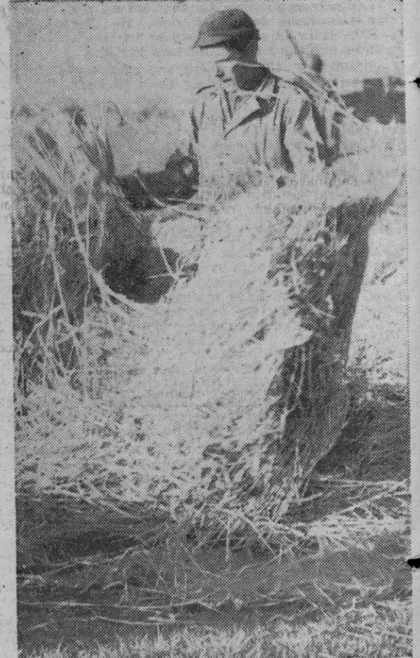
Straw is spread along the soggy German soil before steel is laid for the runway.
