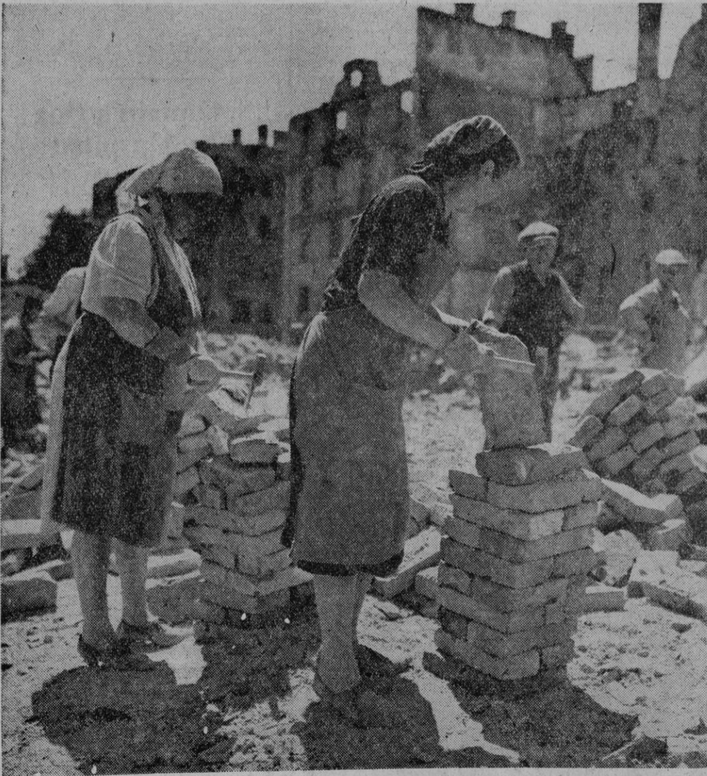
THESE Munich women are chipping bricks, along with male workers. Bombed German cities offer more than enough work for all Germans, regardless of sex. One estimate was that reconstruction in Berlin alone could keep 1,000,000 men busy five years.
