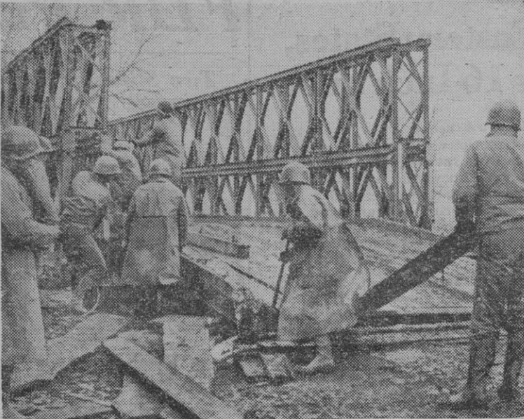
Signal Corps Photo U.S. engineers tighten bolts of a Bailey Bridge spanning a river in eastern France. All along the Western Front, blasted bridges are replaced by spans like these to keep supply routes open.
