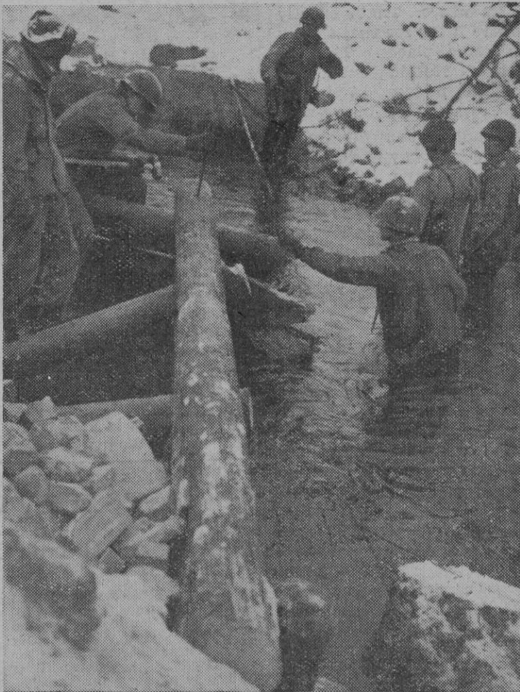
The prevailing thaw on the western Front these days isn't making things any easier for U.S. Army Engineers who are rebuilding bridges wrecked by the Germans when they retreated into the Siegfried Line. Here, men of Co. B of the 171st Engr. Bn., working waist deep in water, erect a foundation on one of the banks of a stream swollen by melting snow.
