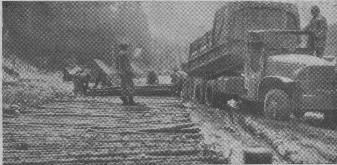
Combating German mud with Yankee ingenuity, engineers of an American infantry division near Zweiff, Germany, construct a corduroy road out of logs felled in nearby Hurtgen Forest.
