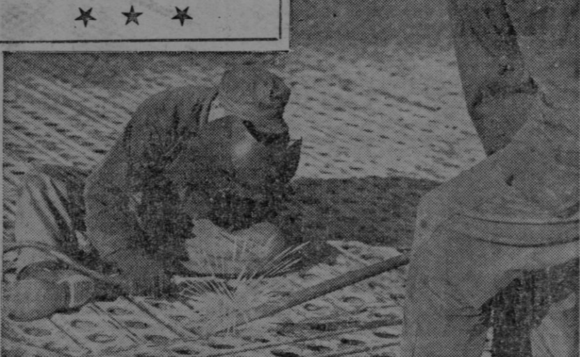
Technicians of IX Engineer Command smooth protruding edges of overlapping sections of steel planking on runway of airstrip. Sgt. A. E. Sellers, left, Danville, Va., handles the welding torch as Sgt. D. U. Barrows, Nashville, Tenn., applies pressure with a steel bar.
