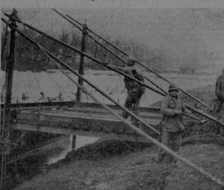
Engineers put finishing touches on the second pontoon bridge across the Roer. The other bridge carried infantrymen across earlier in the drive.
