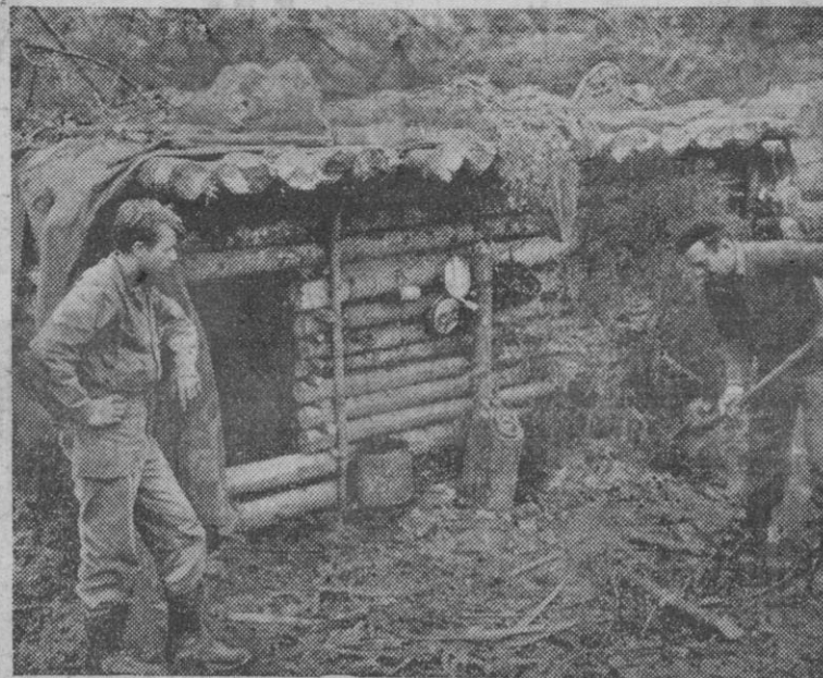
In a windy defile of the Vosges Mountains near St. Die, Pvts. Ernest Madders (left) and Edward Wade, of a Seventh Army field artillery battery, started swinging their axes before snow fell and built this snug log house.
